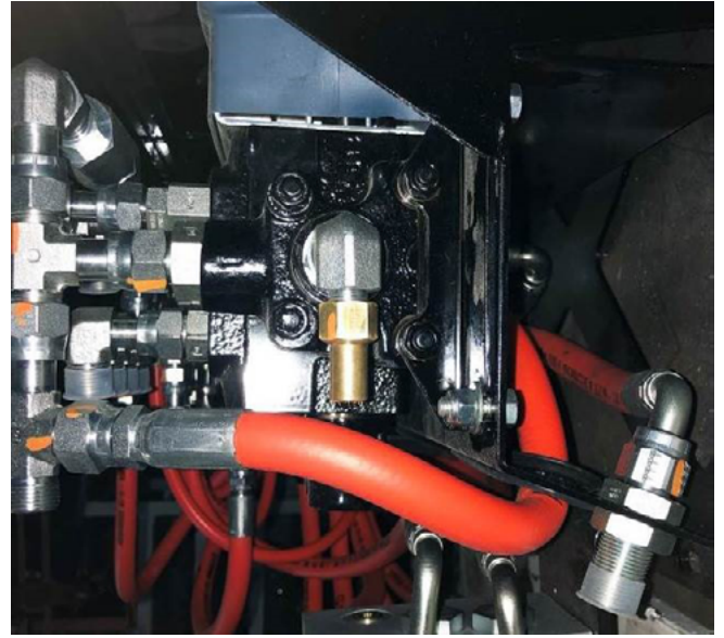
VACUUM CHECK VALVE - UPPER CONTROL
